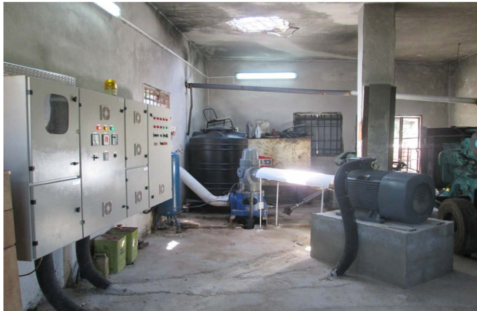
The installed electrical pump at one of the wells
