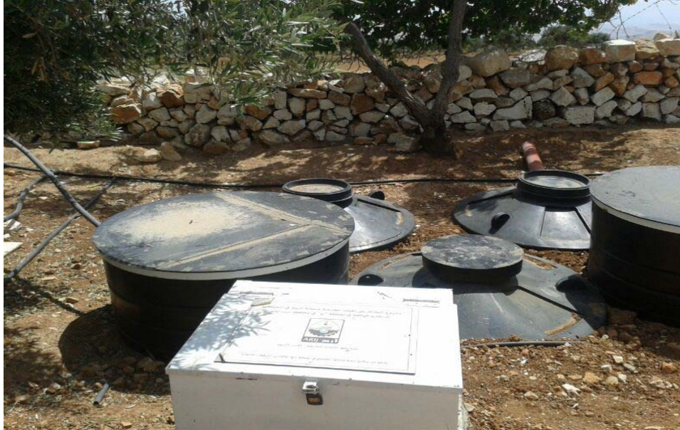
Waste water treatment unit after installation
